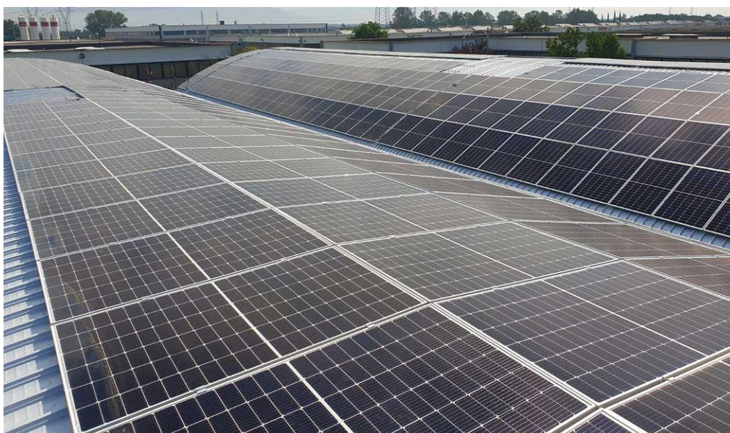
Figure 4-16: PV modules on industrial roofs (source: FuturaSun)
