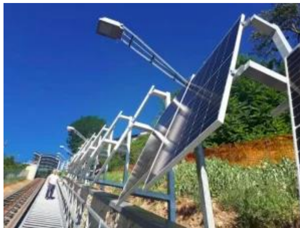
Figure 4-27: PV integrated in street furniture (source: FuturaSun)
