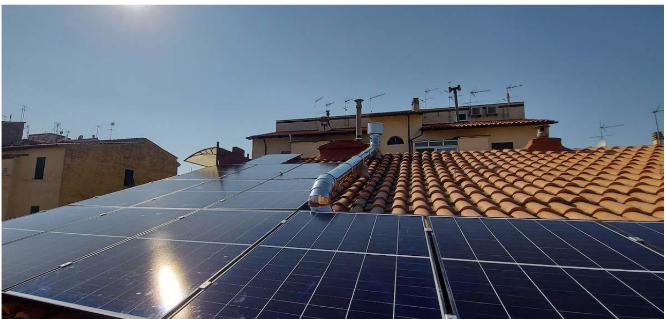
Figure 4-15: ZEBRA modules on residential roofs (source: FuturaSun)
